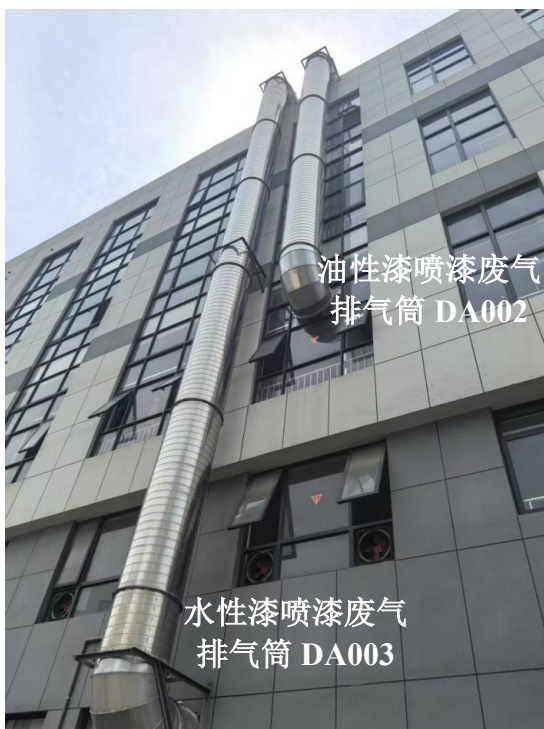
废气排气筒 DA002、DA003
